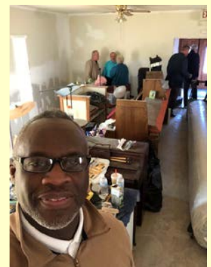
Bishop Coalter, Bishop Davis, and other bishops & pastors touring the damaged churches and seeing the ongoing repairs.
